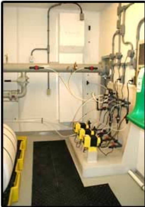
Chemical Feed Equipment
