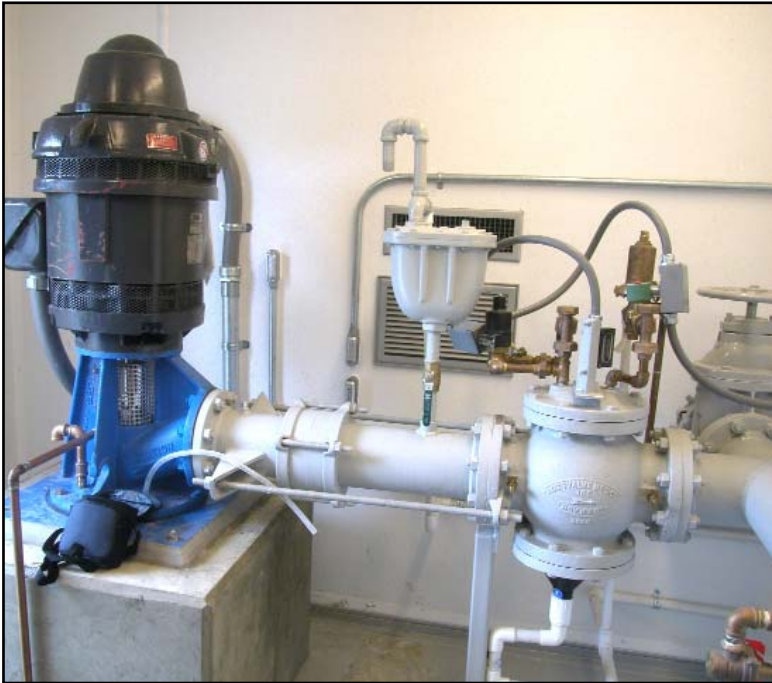
Assembled piping takes water from the well head into the adjacent chemical feed room, all inside a factory-built station delivered complete to the jobsite.
