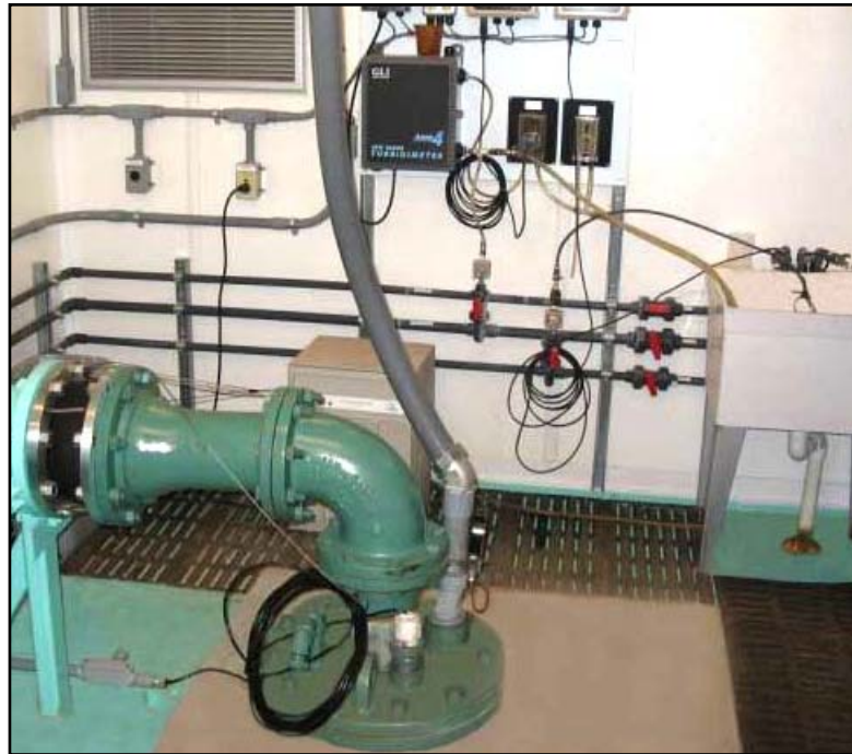
Well starter, feed rate controllers, residual analyzer, turbidimeter, sample sink and level sensor are built into a submersible well pump, water treatment plant.
