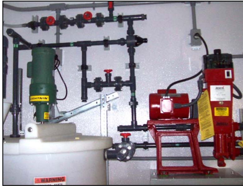
A pH Adjustment System with mix tank, feed pumps, piping and control system is built into one room of a factory-built, well head treatment facility.
