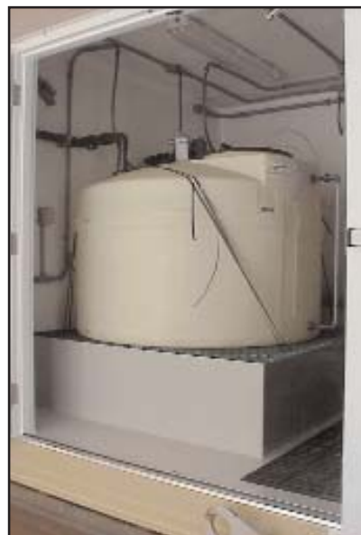
Chemical storage tank with containment structure.
