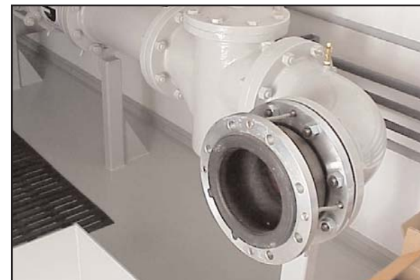
Connection point for well pump.
