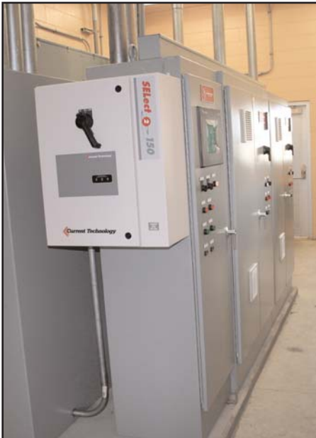
Remote mounted VFDs, distribution equipment, and PLC controls also provided by EFI.
