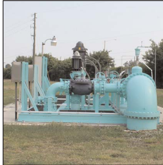
View of the discharge head end of skid pump station.
