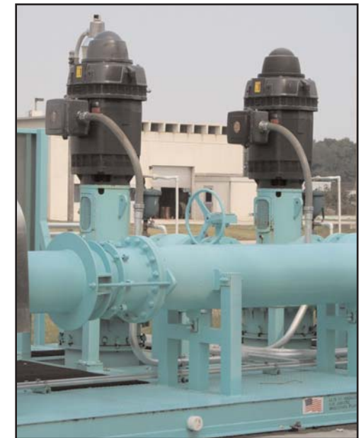
Vertical turbine pumps shown here with discharge piping and electrical equipment building in the background.
