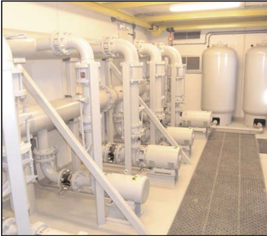
Station interior with pumps and hydro. tanks, header pipes, and valving and bridge crane.
