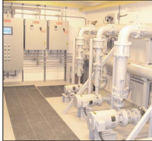
Station interior with PLC based controls and telemetry in the EFI Water-Shed building.
