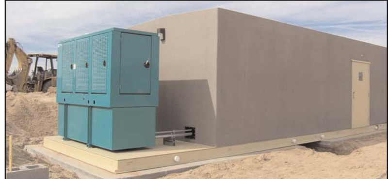
Exterior of pump station with stand-by generator all on factory-built steel skid.
