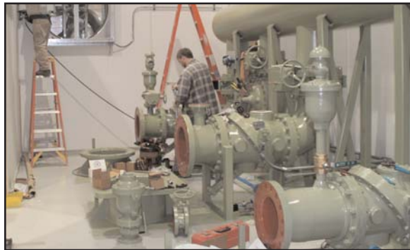
Shop assembly of mechanical components including pump check valves and isolation valves and the discharge header.
