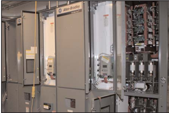
4160 Volt Motor Control Center being assembled. Each half of the building had its own set of pumps and controls with separate power feeds for complete redundancy.
