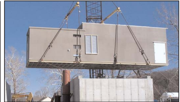
First of two building halves being lifted and placed on top of the intake structure. The low roof portion is the electrical room and is separate from the pump room.
