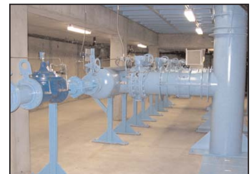
Basement view of piping for the turbine pump barrels.
