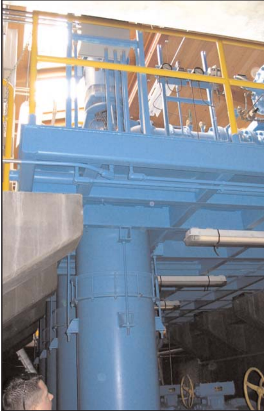
View of skid station above and piping in the basement.
