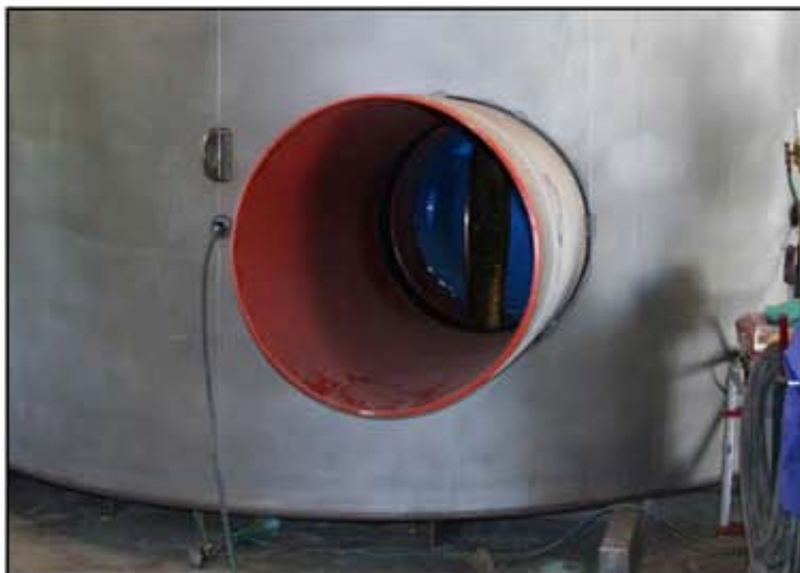
This picture shows the piping coming through the capsule sidewall and tack welded into place prior to the inside and outside seal welding operation. The transmission pipe at the capsule shell weld joint has a 2" thick steel sleeve welded over it where it passes through the capsule wall; this sleeve pipe lining is attached prior to fusion bonding the pipe serves as a heat sink to keep the capsule seal weld heat from burning the fusion-bonded epoxy.
