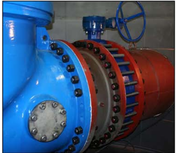
This picture shows the 36" valve assembled into the transmission piping with the inlet-side isolation, wafer butterfly valve.
