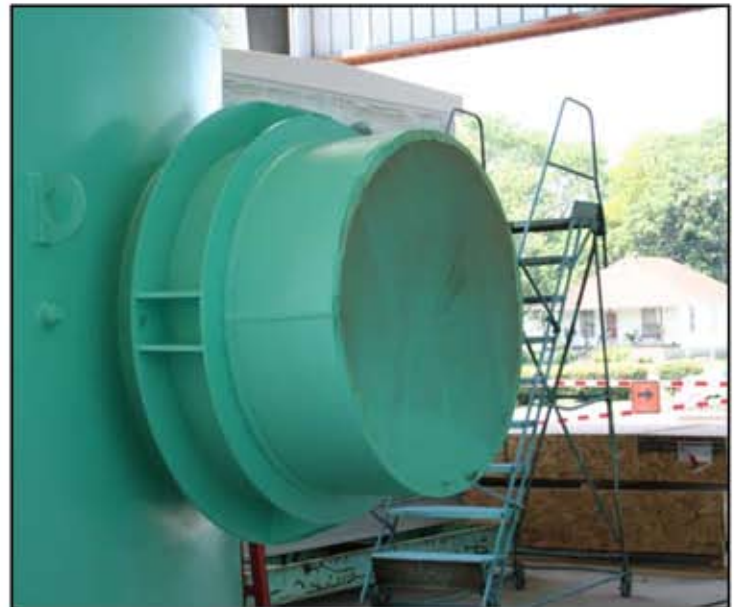
This picture shows the AWWA-M-11 restraints system built onto the transmission piping.
