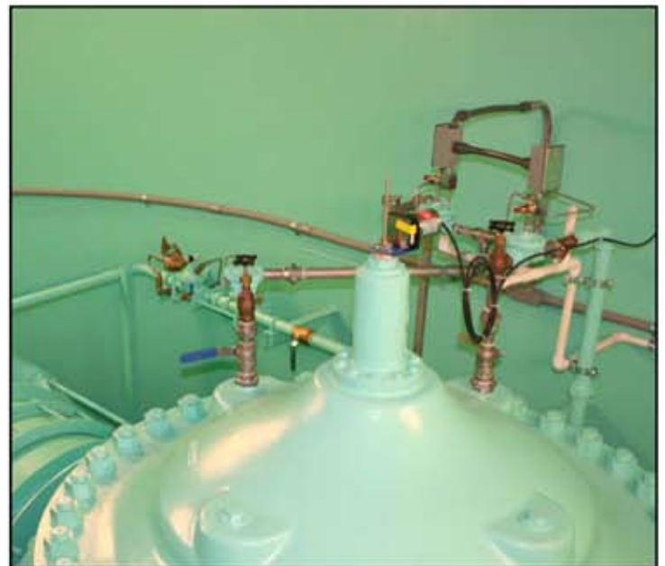
This picture shows the pilot piping and valving including the pilot control water supply line from the pressure tank.
