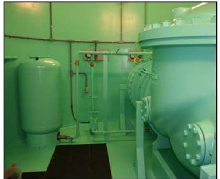
This picture shows the pilot water system tank, pump and piping. Behind the 36" control valve is shown the breakaway coupling included to facilitate valve withdrawal if ever required.
