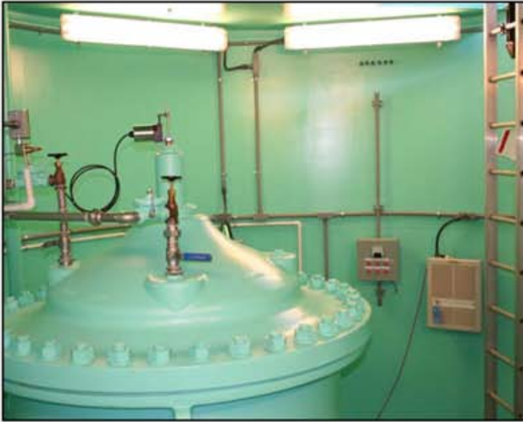
This picture shows the cover chamber and the tank wall welding along with the ladder to the manway hatch, the heater and the cathodic protection system, anode test station.
