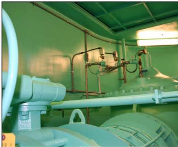
This picture shows the tank top sheet with a steel, reinforced 7' x 7', equipment hatch above the valve for valve withdrawal and for lifting the dome off the valve for servicing the internal parts when required.
