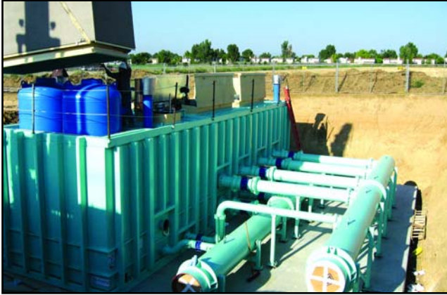
31.6 MGD Booster Station Thornton, Colorado
