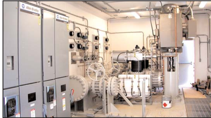
Interior view with pumps set.
